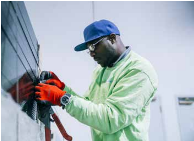
A worker with a business named Solar Liberty installs solar panels in Buffalo, New York. NAFTA's replacement should encourage investments that create good jobs and clean energy. By contrast, the deal should not offer incentives to invest in fossil fuels or other businesses that are incompatible with a just transition to a clean energy economy. Photo: Stephen Yang
