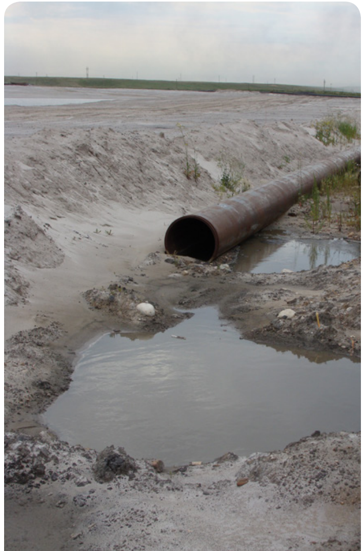
Pipelines bring the risk of spills and contamination.
